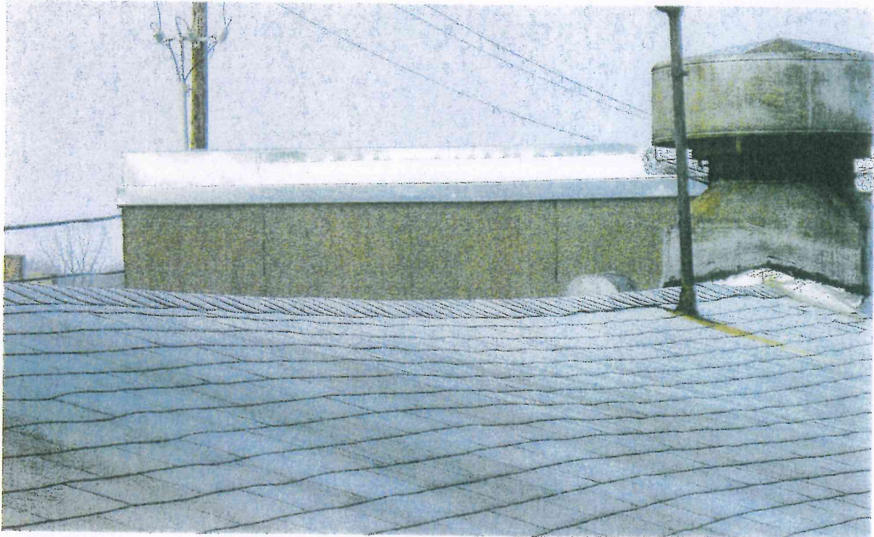
Photo 48 - . . . especially evident at the peak of the gable.
