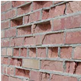
Excessively deteriorated brick
