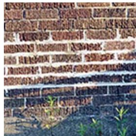
Inappropriate mortar work
