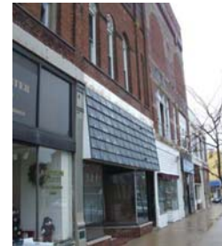
Inappropriate materials and use of Mansard roofing.
